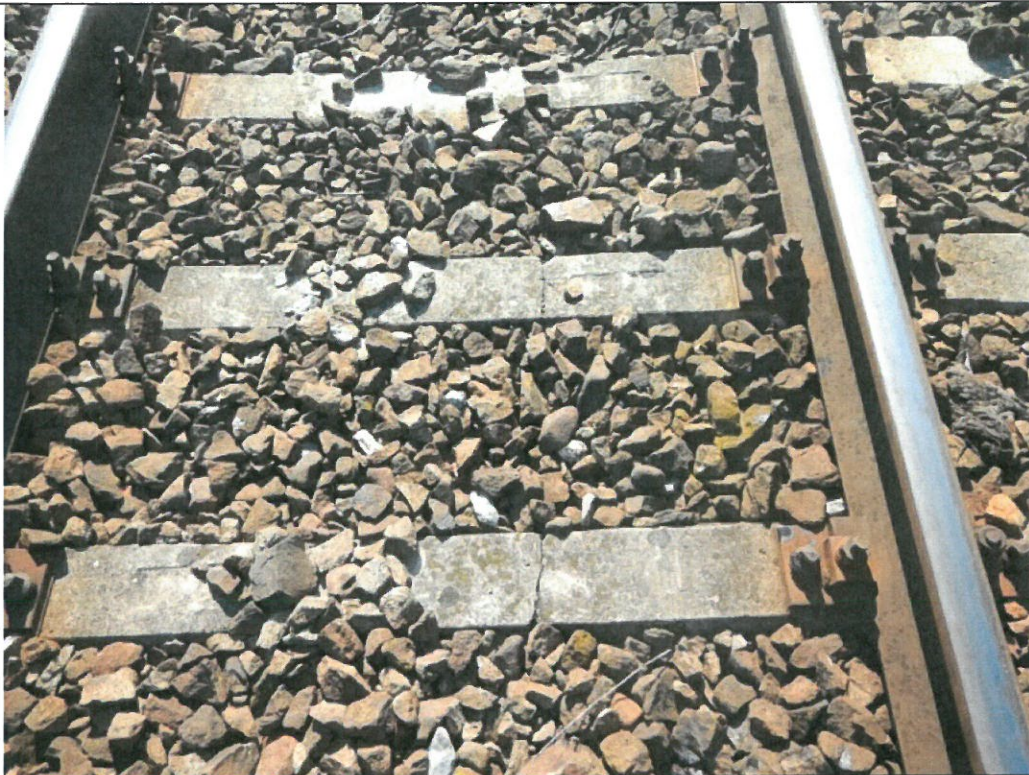
Traverse de beton consecutive cu fisuri transversale
