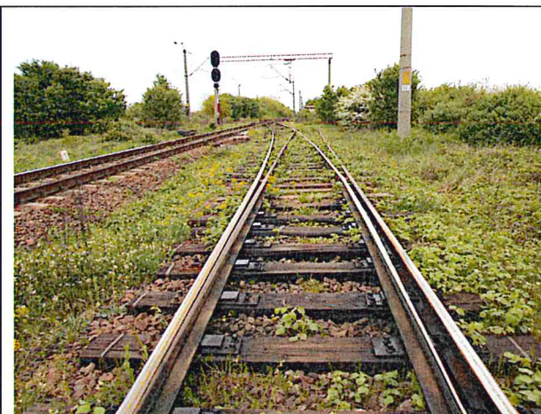
Km 46+100 – prisma caii acoperita de vegetatie, santuri colmatate
