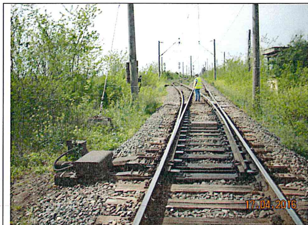
Km 497+300 – traverse de lemn crapate si fisurate, lipsa santurilor
