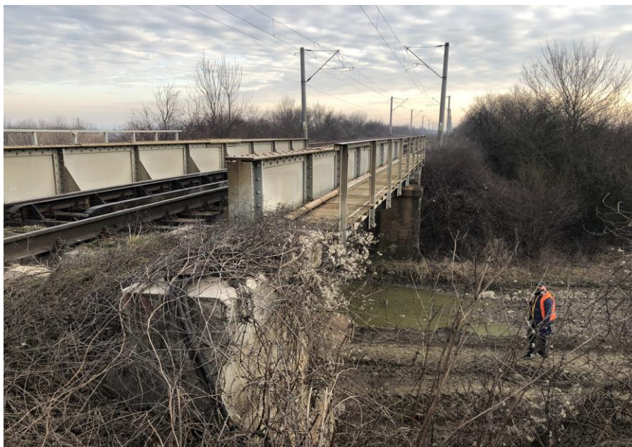
Pod km ex. 22+243 – Prelu degradat
